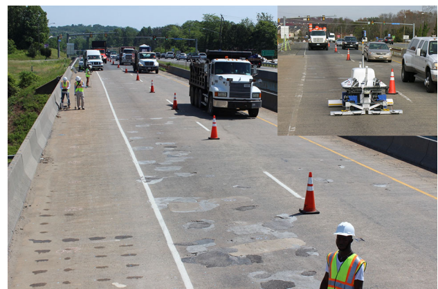
Fig. 10 View of the deck and RABIT data collection on the Haymarket Bridge
