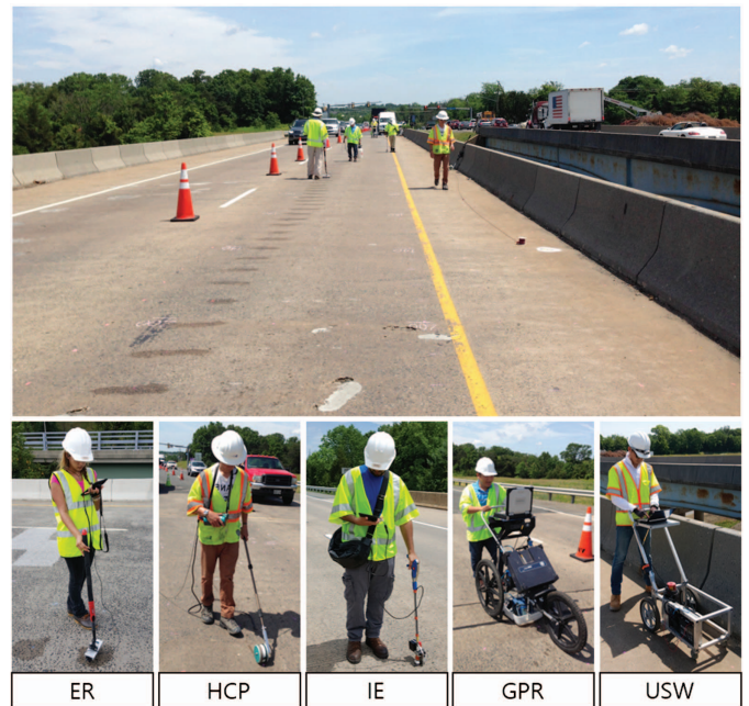
Fig. 2. (Color) Nondestructive evaluation data collection on the deck of the studied bridge.
